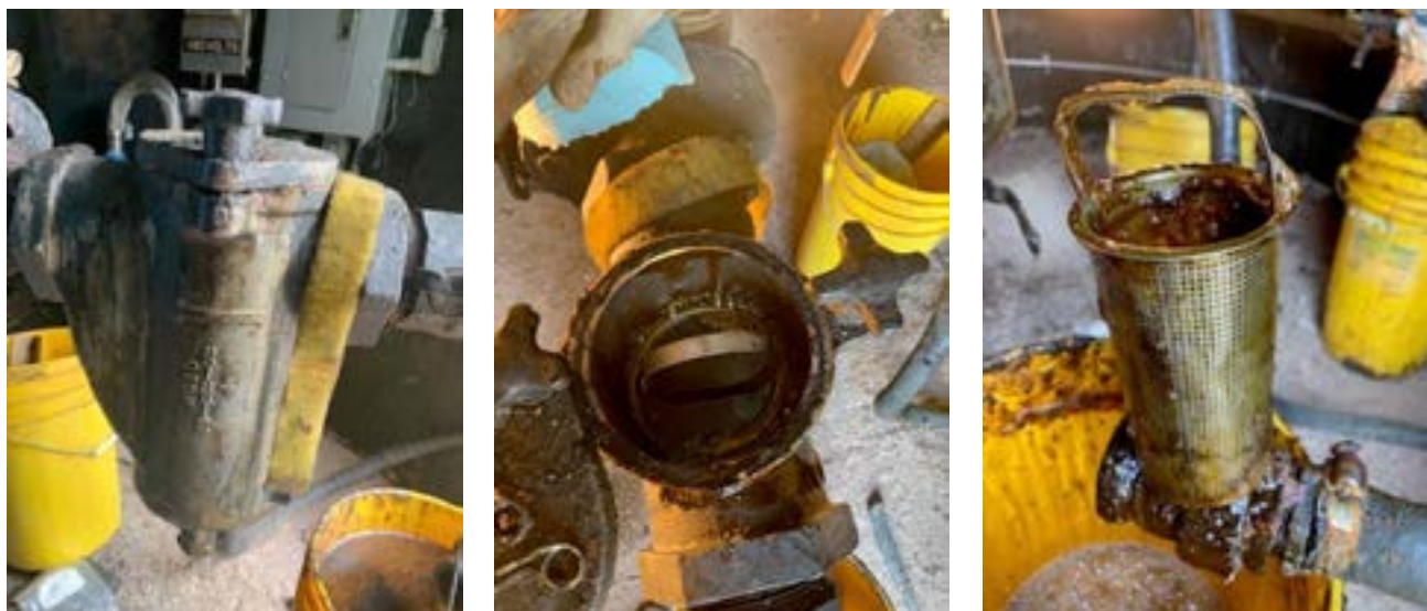
Figure 10. Enclosed stainless steel basket strainer (left), exposed basket strainer showing the strainer inside the cavity (center), external view of extracted strainer (right). Source: J. Lechman, J&R Consultants, Ltd., Winnipeg, MB, Canada.
